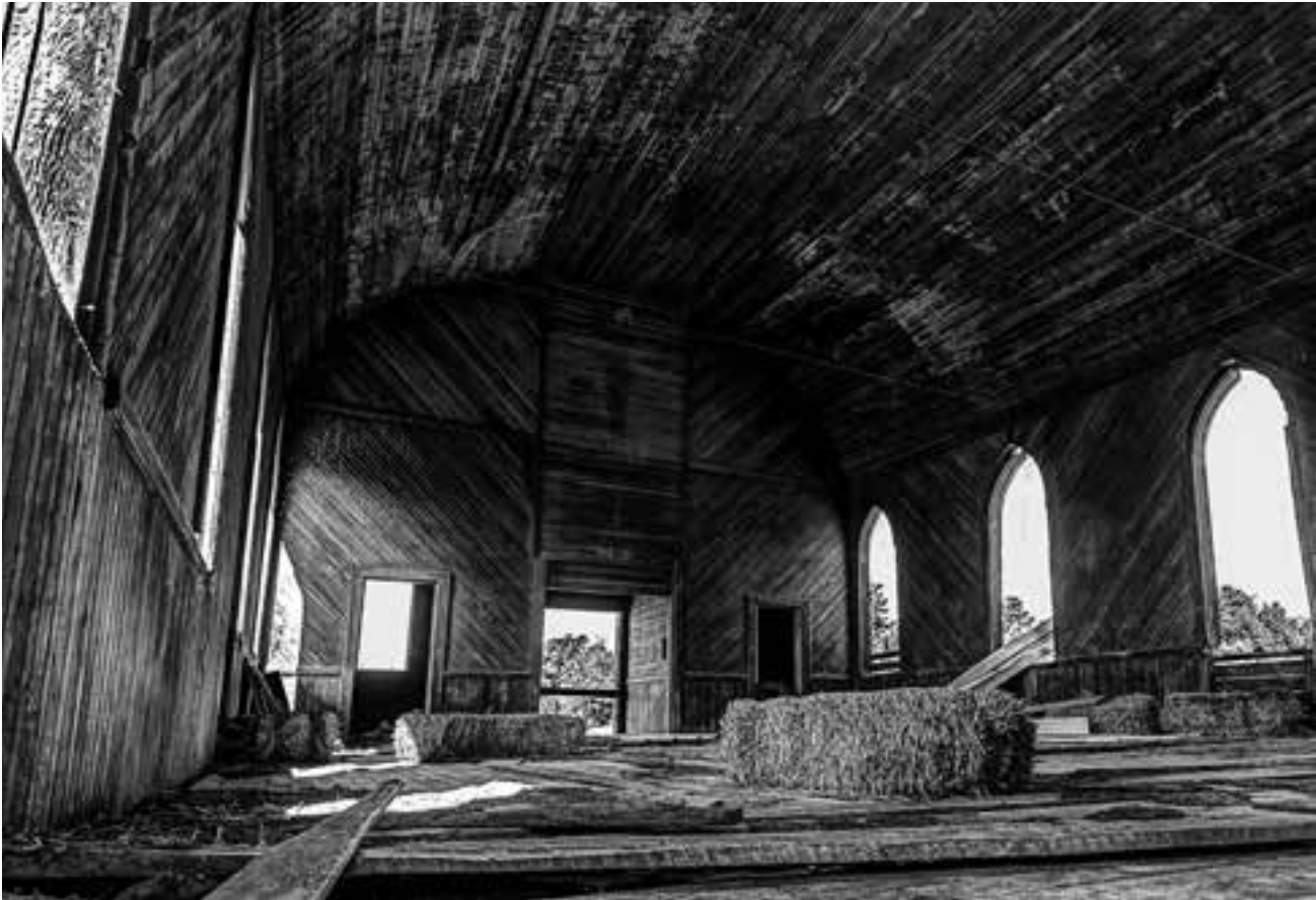
Restoration underway inside the Locust Grove Church on the Wasco-Celilo Highway in Locust Grove, Sherman County, Oregon. The project has been plagued by vandalism.
